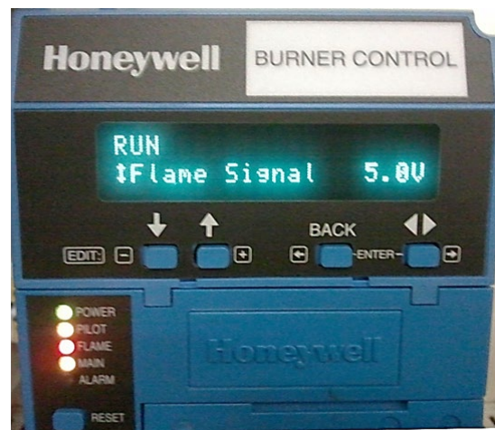
Fig 9 Honeywell Burner Control
